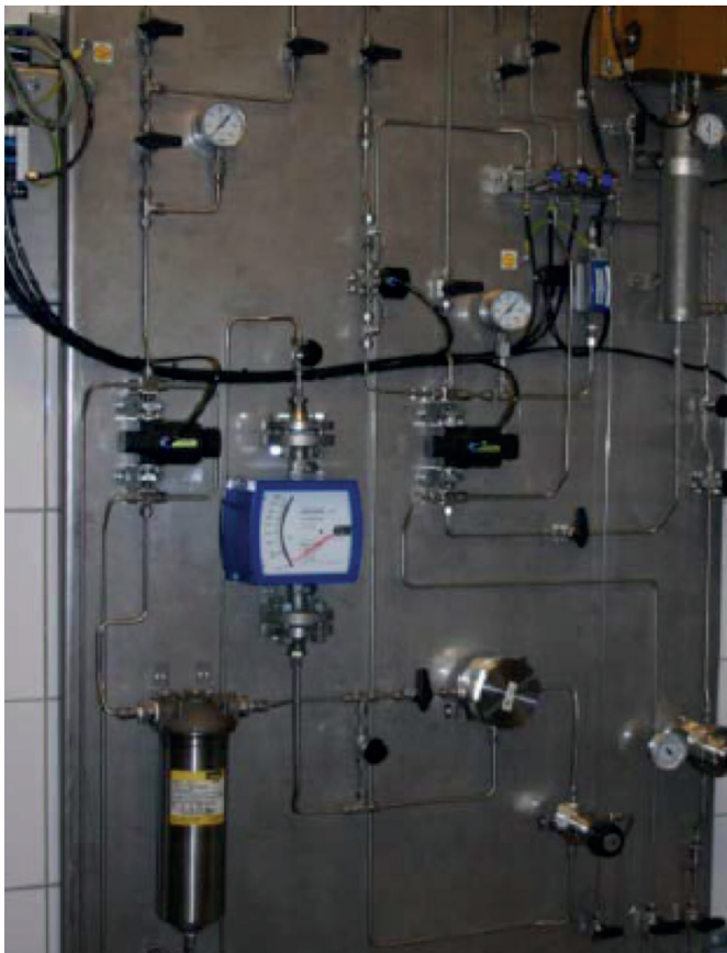
Sample conditioning and sample flow-cell panel with fastloop filter, h /exchanger and coalescer.
